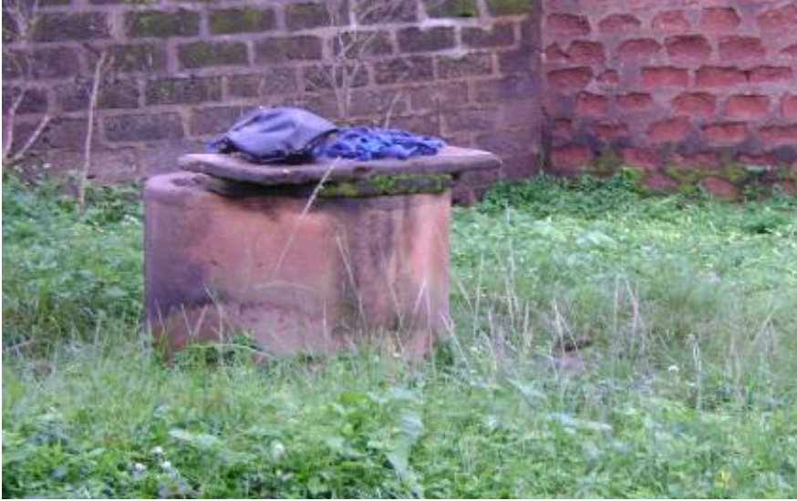
Figure 4: A well with rotten wood slab
