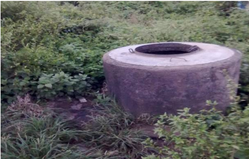
Figure 5: A well which metal cover had rusted and fallen off.
