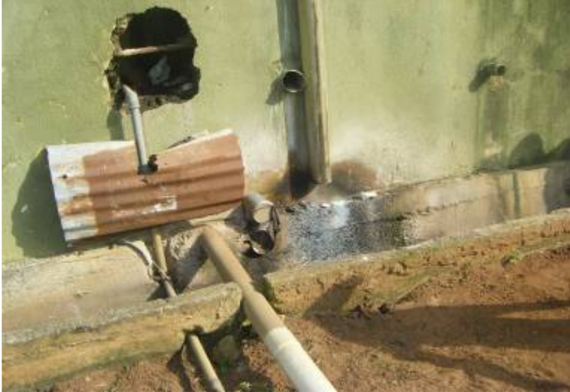
Figure 1: A section of the water pipe supplying water to Hall B positioned above a sewer.
